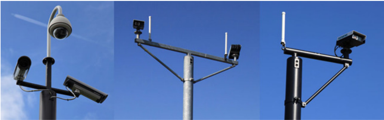
Figure 1: Pole mounted CCTV arrangements
