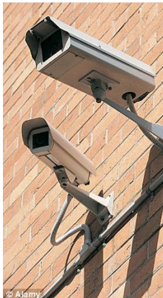
Figure 2 – Building mounted CCTV arrangements
